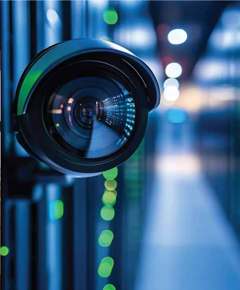
24x7 CCTV Surveillance
